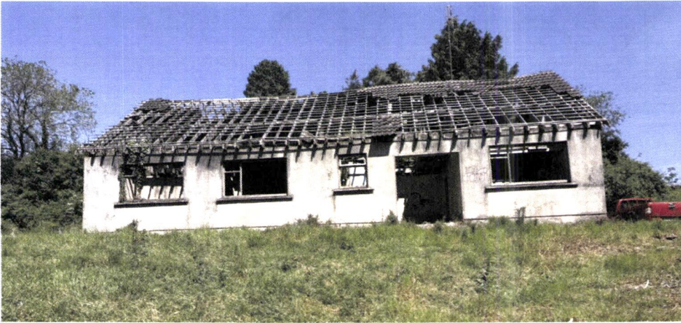
Fig. 6: Photograph of the existing dwelling structure with its windows and roof tiles removed for delayed maintenance (3)
