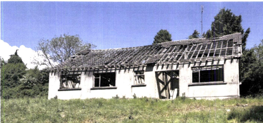
Fig. 5: Photograph of the existing dwelling structure with its windows and roof tiles removed for delayed maintenance (2)
